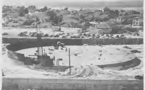
STEEL FLOORING is laid on the sand, and welded to the first row of plates in the wall—the first "shell course." VLOER DI staaí ta worde poni ariba e santio, y gwerdo na e promer fila di plachi den e muraya — e promer "shell course."
